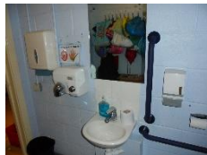
Mirror and paper towel dispenser too high and grab bar missing from side of sink
